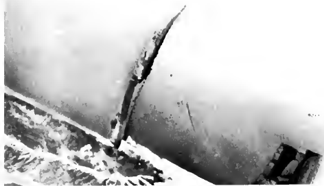
Photo 3. Second Los Angeles Aqueduct. Compression failure in 76-inch Saugus pipeline at mid-slope on north side of Terminal Hill. Note that saddle pier at lower right is displaced downhill as it moved with hill slippage. Los Angeles Department of Water and Power photo.
